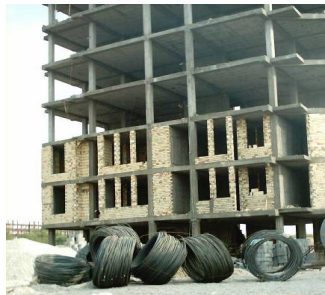
Fig. 8. Lack of restrictions of infill and improper portioning of frame elements
