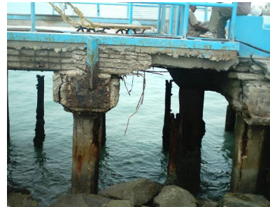
Fig. 7. Devastating condition of seaport
