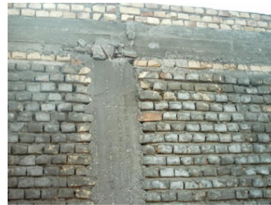
Fig. 9. Lack of integrity in concrete ties connection
