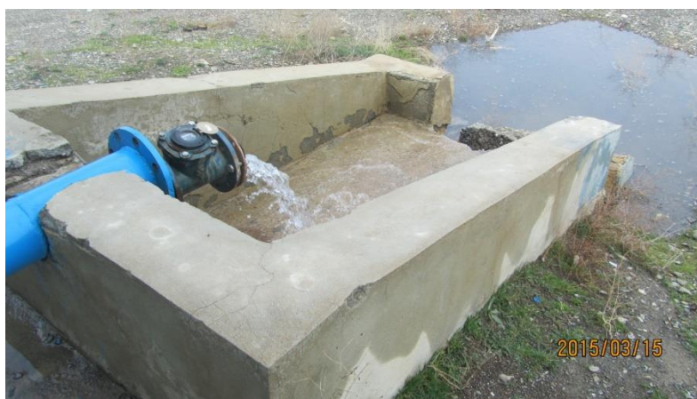
Fig. 3. Created leak in well number W12.
