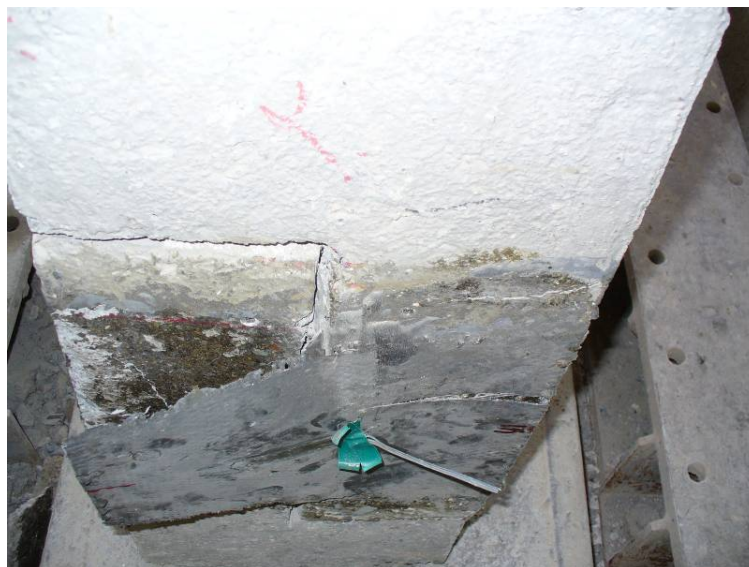
Fig. 4. Debonding failure pattern of the strengthened push-off specimen PCRC3.
