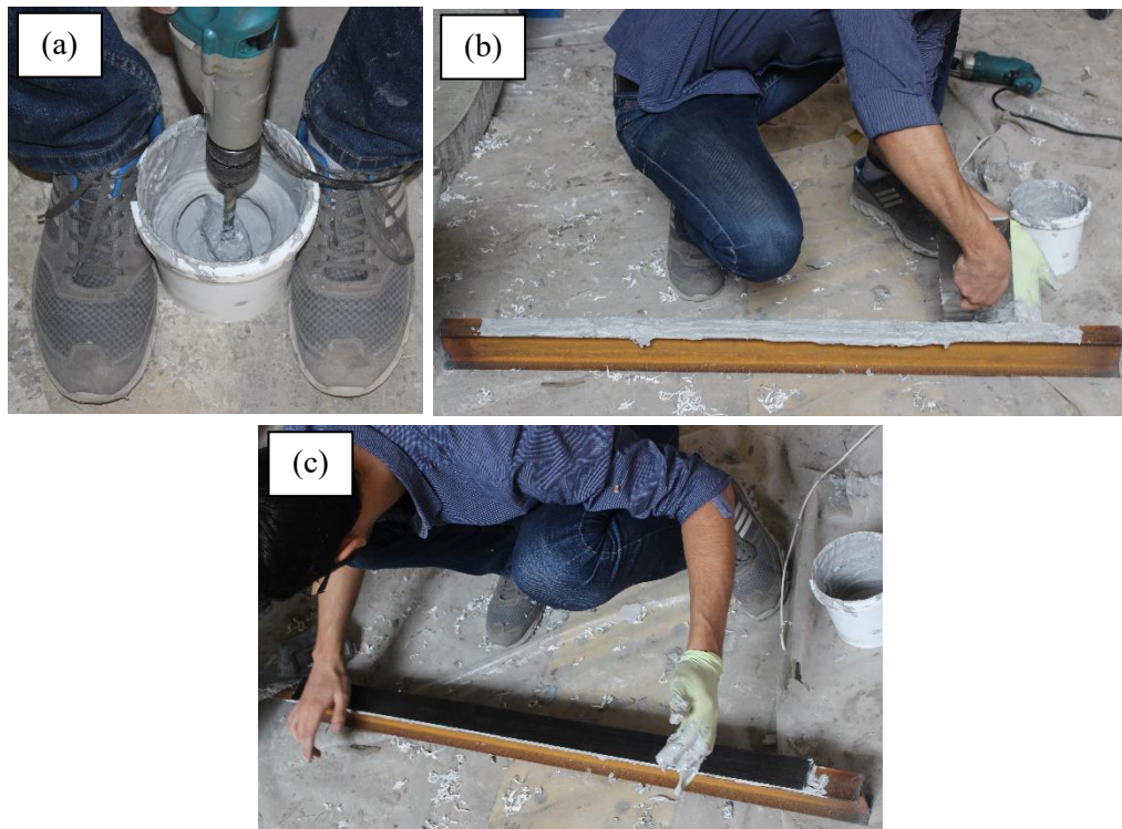
Fig. 3. (a) Mixing two components of adhesive. (b) applying the epoxy adhesive on the flange surface. (c) attaching the carbon laminate to the steel beam.
