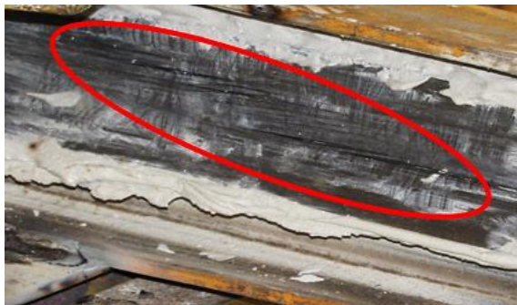
Fig. 15. CFRP parallel cleavages oriented at almost 45 degrees in beam S-IPE100-R.
