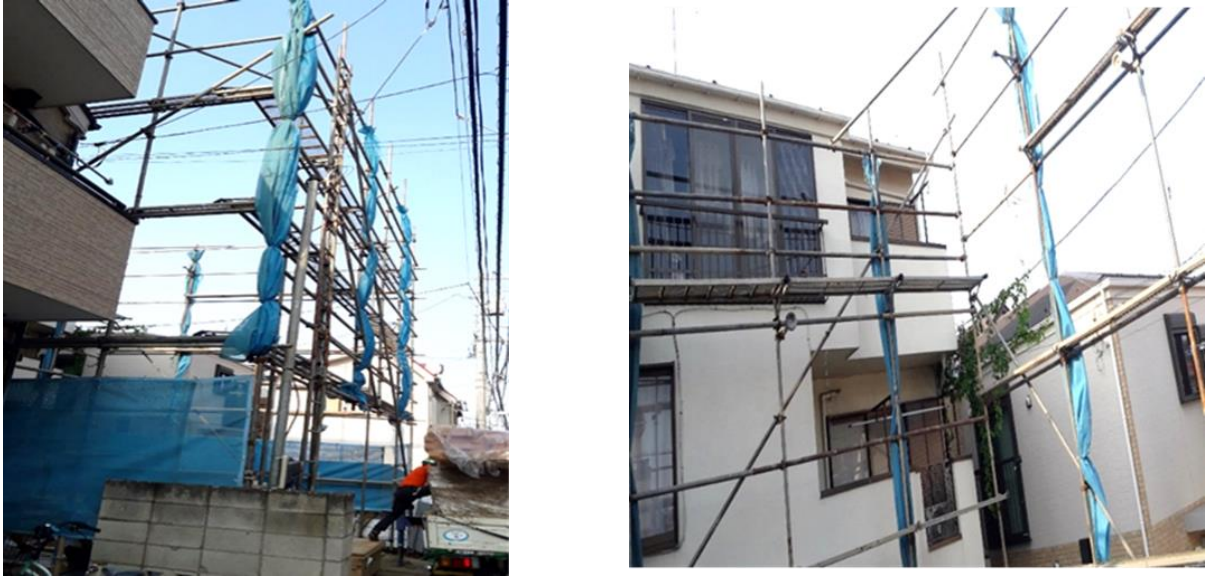
Fig. 3. Absence of scaffold insulator (left) and guard rails (right).
