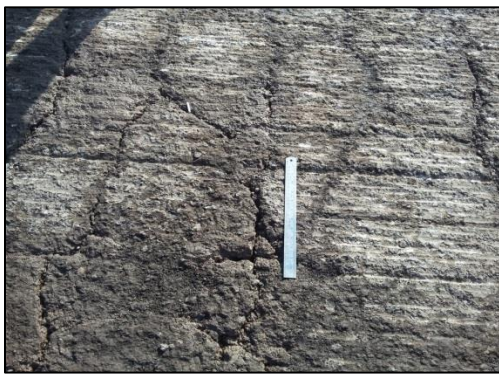
Fig. 6. Reflective cracks after 7 cm scraping and cutting.
