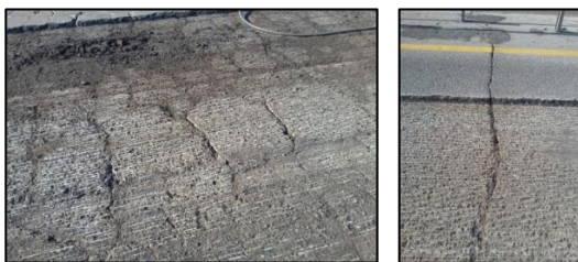
Fig. 7. Reflective cracks after 10 cm scraping and cutting.
