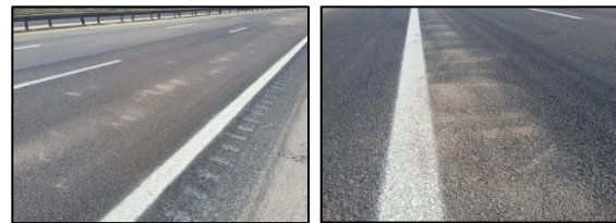
Fig. 9. Section 2 of 23 km, movement of mud from the lower layers to the upper layers after precipitation.
