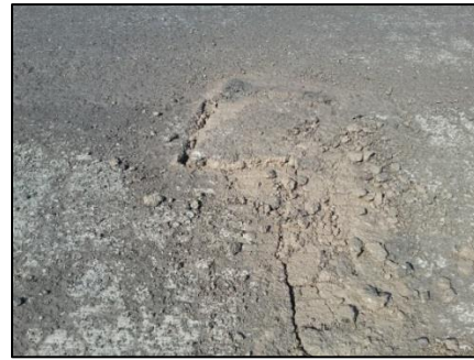
Fig. 12. Section 2 of 22 km, removal of mud from the cracks after cutting the top layer.
