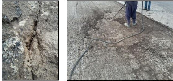
Fig. 11. Section 2 of 23 km, removal of mud from the cracks after cutting the top layer.
