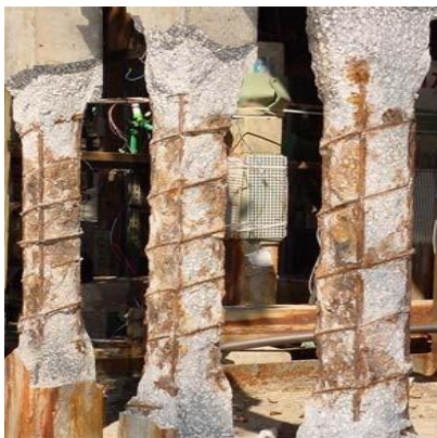
Fig. 1. a picture of a deteriorated rebar due to corrosion.
